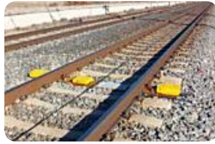
Hotbox detection devices installed on the railway track photo: SCIL AG
